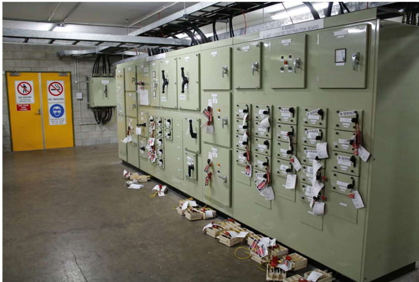
Figure 123 Unit C4 DC switch room
