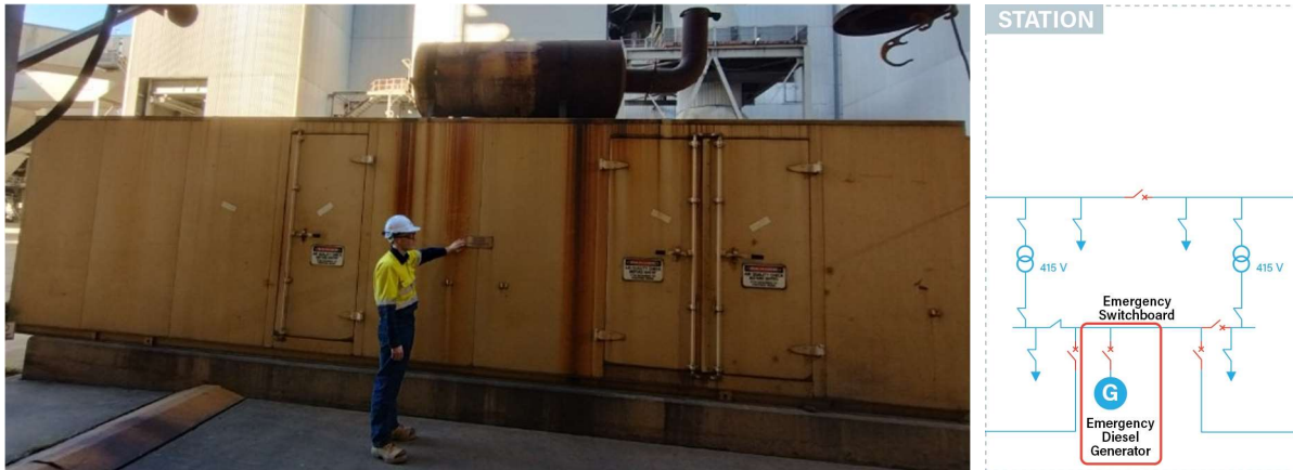
Figure 59 Emergency diesel generator
