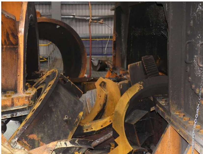
Figure 38 Damage between the generator and the LP turbine
