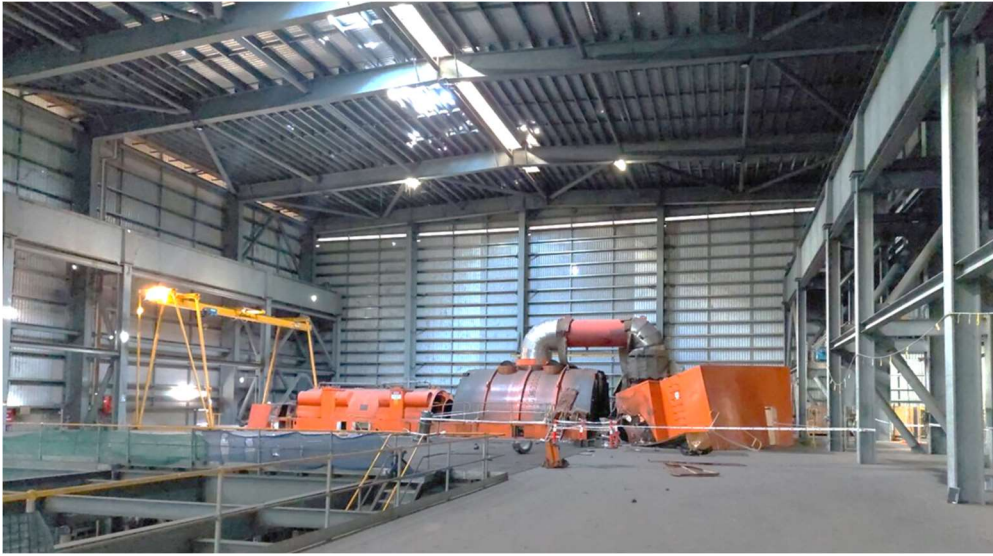
Figure 124 Post-incident Unit C4 in the turbine hall
