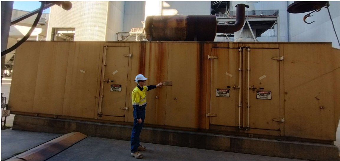
Figure 21 Callide C emergency diesel generator
