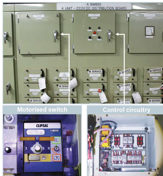
Figure 20 Unit C4 automatic changeover switch
