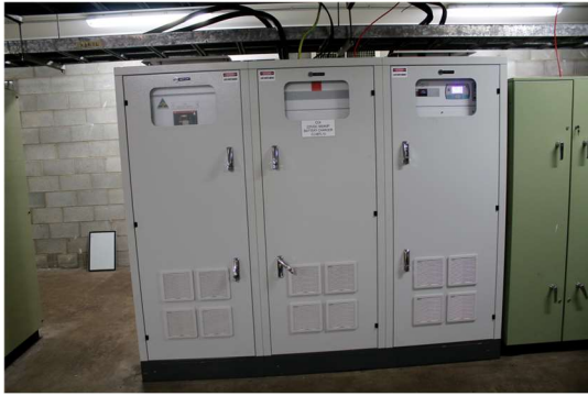
(a) Unit C4 battery charger
