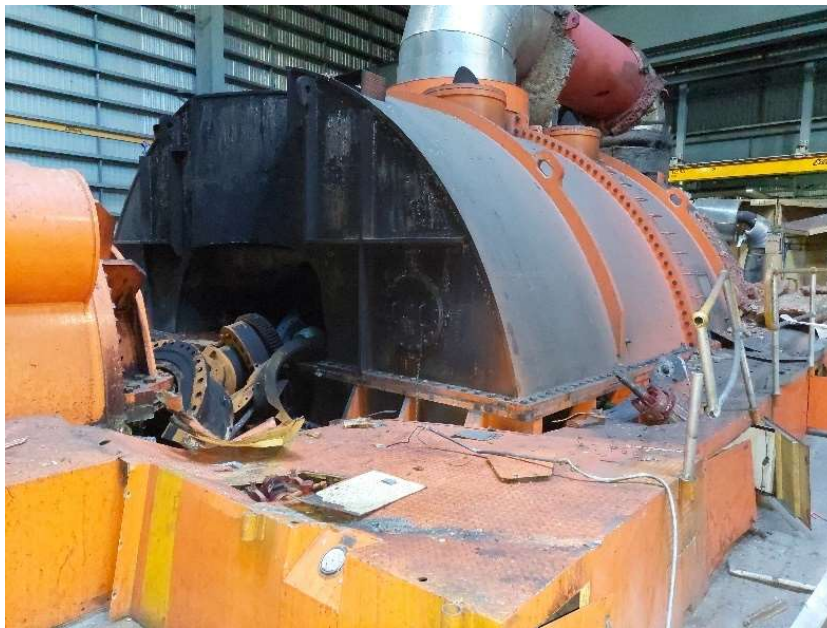
Figure 41 Heat damage to LP turbine casing
