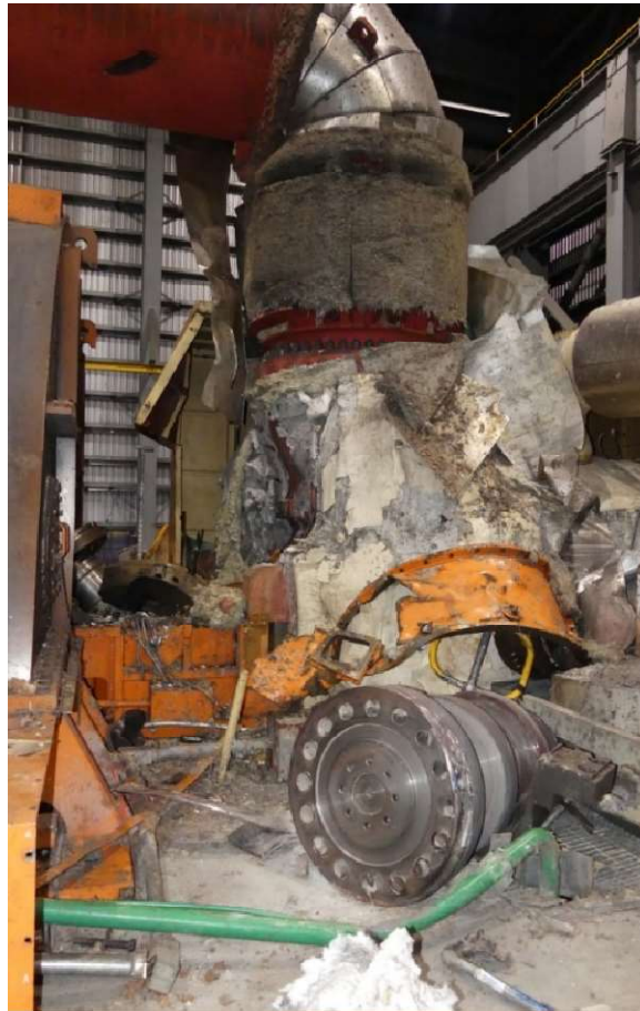
Figure 39 Damage between LP and HIP turbines
